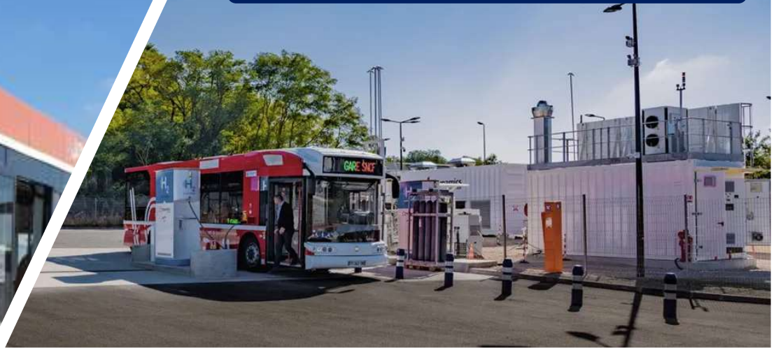
AuxHYGen - LINE 1 | Auxerre H2 PRODUCTION ON SITE
